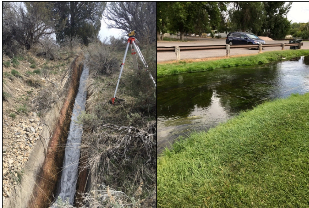
Fig. 4. Many canals in Utah were constructed along very steep slopes. In the left-hand photo, the Mt. Nebo Canal (Site UC2, see Table 4a) descends along a slope S = 0.3669 . In the lower part of the canal wall, the concrete finish has been stripped away to expose the rough aggregate underneath. In the right-hand photo, the Lions Park Canal (Site UC11, see Table 4a) is an earthen canal with banks of grass and dense weeds, descending at a slope S = 0.0052 .
