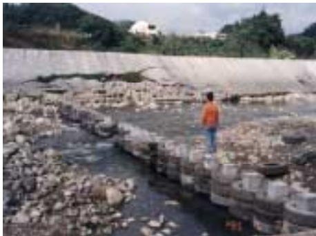
Photo 3. Tire weir with opening
