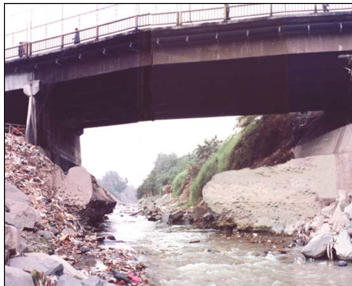
Figure 2. View showing the bed level in 2001. Notice that the river flows underneath one opening. Also notice scour in the right bank (left) and leftovers of a remedial work.
